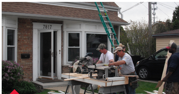
The Residential Sound Insulation Program (RSIP) was established in 1995, and has sound-insulated more than 21,000 homes near O'Hare and Midway. A new mitigation plan will address issues some homes have experienced with odorous or mechanically defective RSIP windows.
